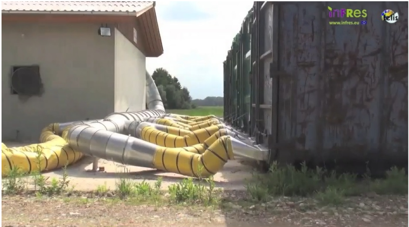
Air ducts supplying containers with heat
